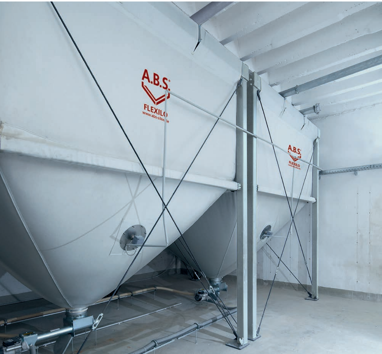
Storage cascade comprising Flexilo Maxi (30 t) for 100 kW pellet heating system in a grammar school
